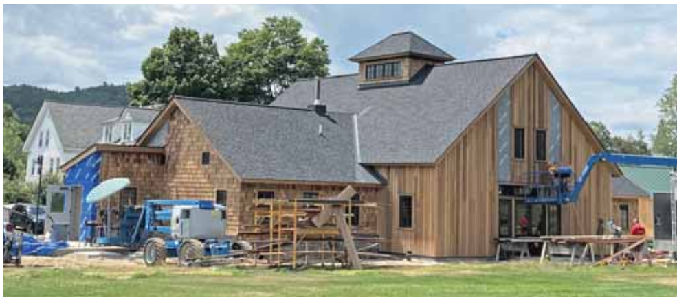
The Proctor Woodlands Building is nearing completion. The final project in the $40M+ Campaign for Proctor, the Woodlands Building will serve as a science teaching space and gateway to Proctor's 2,500 acres of woodlands. The timber frame construction of the building utilizes timbers harvested on Proctor's land near Elbow Pond. Caption and photo: Scott Allenby
